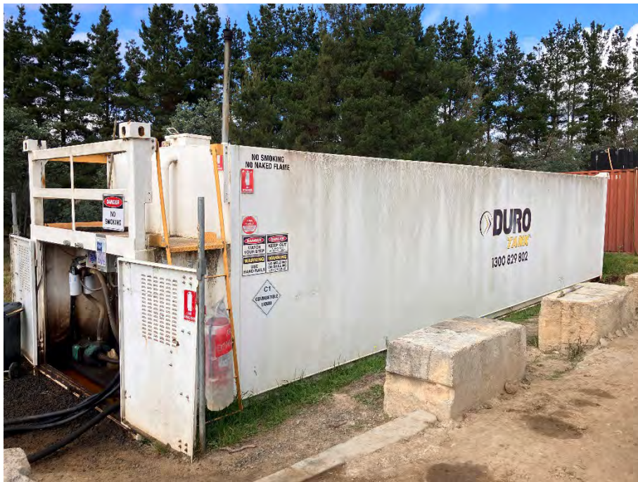
Photo 18: Self-bunded diesel storage tank, looking southeast.
